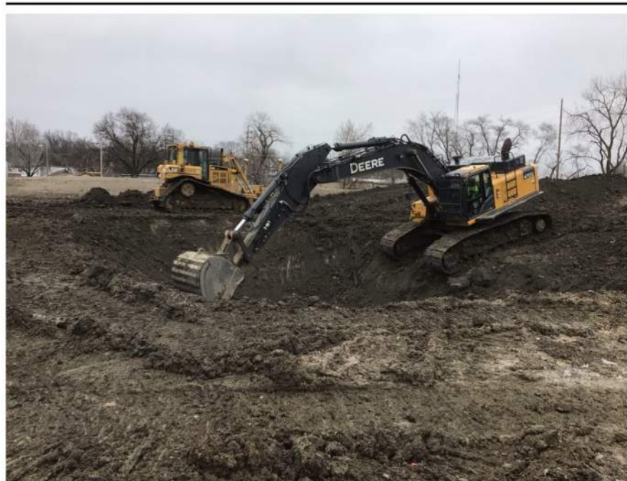
Excavation and earth moving operations for large sewer overflow structure at Mary Avenue.
