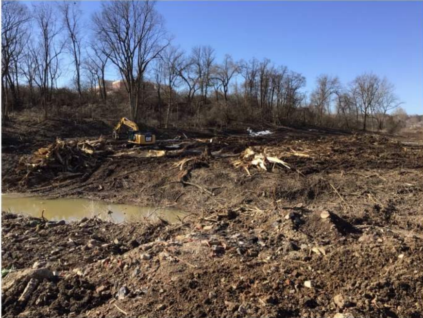
Tree removal operations at Parcel 93 for accomplished clearing, grubbing, and stripping work.
