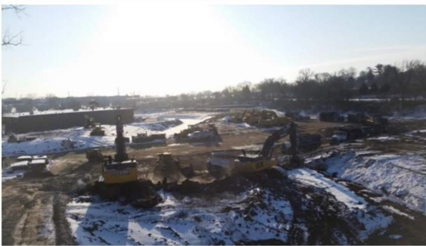
Mass excavation and haul-off operations at Parcel #65 for floodplain redevelopment and restoration.
